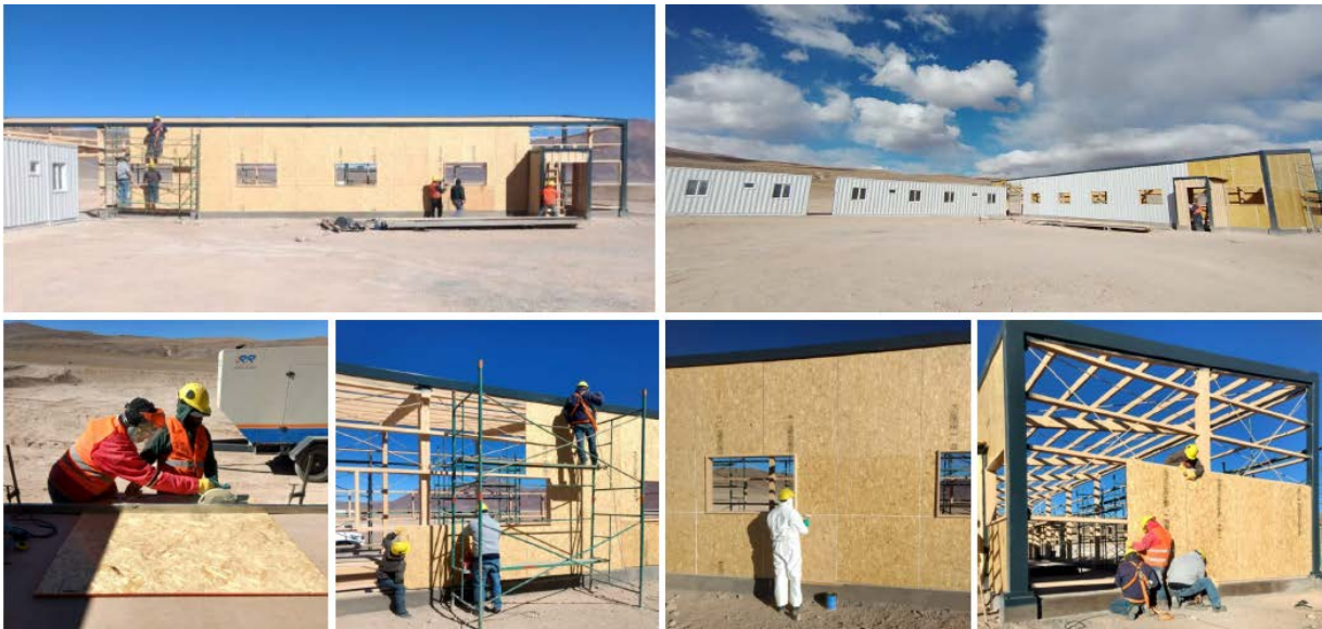
Figure 2. Rincon Lithium Project – 2,000tpa Operation Site Works in Progress (camp construction works)
