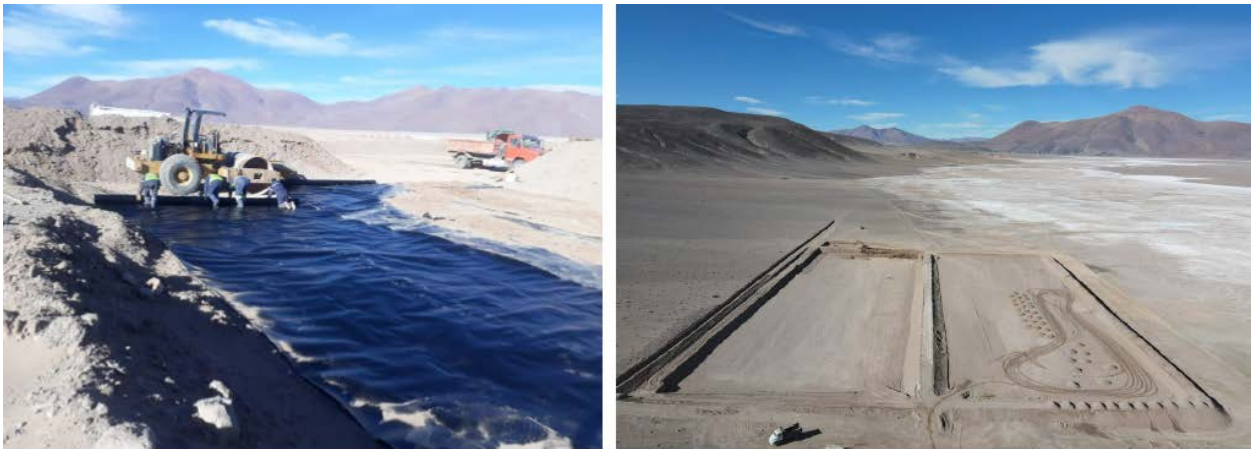
Figure 3. Rincon Lithium Project – 2,000tpa Operation Site Works in Progress (plant settling ponds works)
