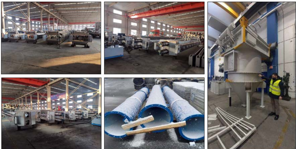
Figure 3. Rincon Lithium Project – 2,000tpa Operational Equipment (Dryer & Press Filters)
