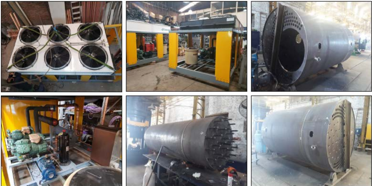
Figure 2. Rincon Lithium Project – 2,000tpa Operational Equipment (Boilers & Coolers)
