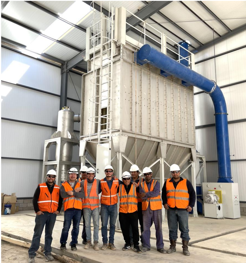
Figure 3. Rincon Lithium Project – Installed Evaporator/Dryer
