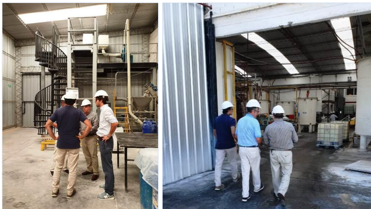
Figures 4-5. Rincon Lithium Project – Pilot Plant Lithium Carbonate Production Operations, with plant visit by new Salta Mining Secretary
