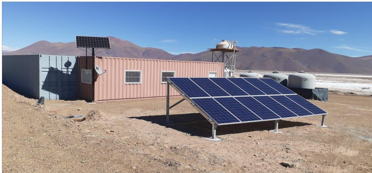
Figure 2. Rincon Lithium Project – Installed Solar Panels Providing Power on Site
